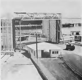
THE REFINERY'S new main entrance will officially open Tuesday, June 4. Lago police will occupy the foremost section of the new gatehouse here. The employee walkway will be between the fences.
